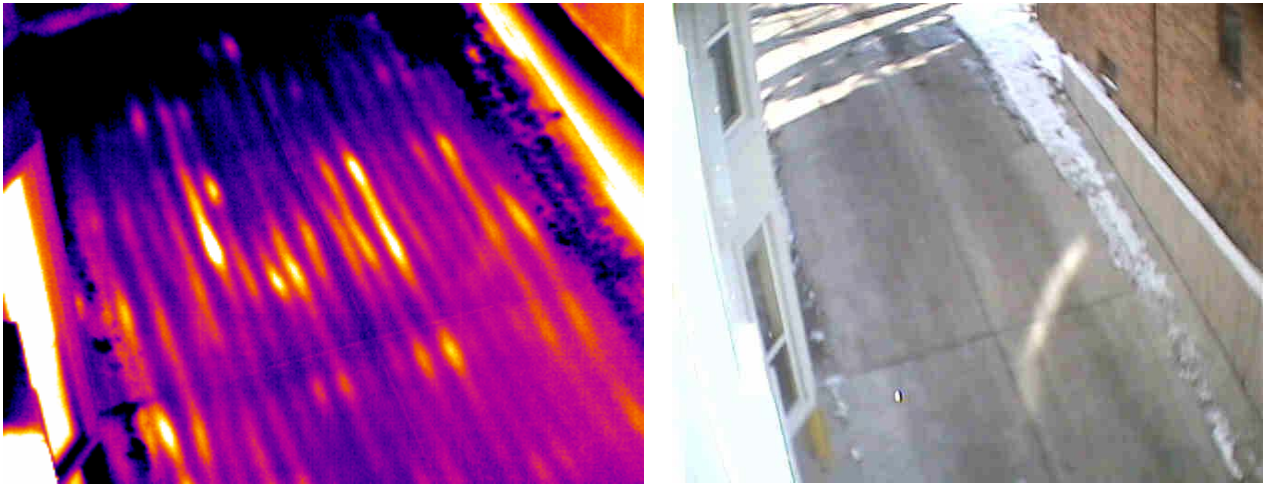
Figure 6. Note differential heating of lines indicating multiple variances in radiant heat line depth below the surface of the concrete.
